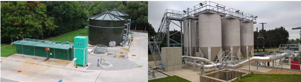
Figure 3-5: Plant required for permit less than 1 mg/l – chemical dosing plant, tertiary sand filters and sludge tanks (pumping station not shown)
