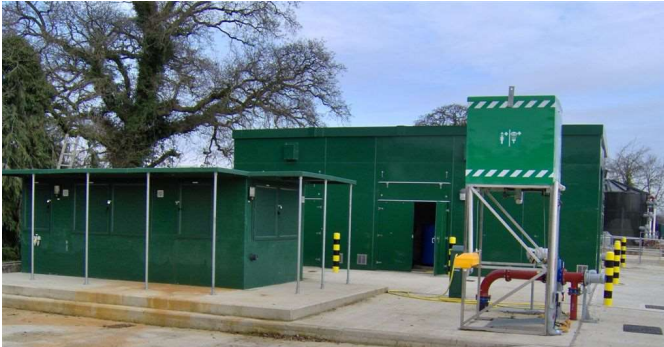
Figure 3-4: Chemical dosing plant for 1 mg/l P permit
