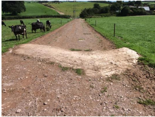
Resurfaced cow track with cross-drains installed. Funded by the Somerset Rivers Authority / FWAG-SW Hills to Levels project. (Photo credit: FWAG-SW)
