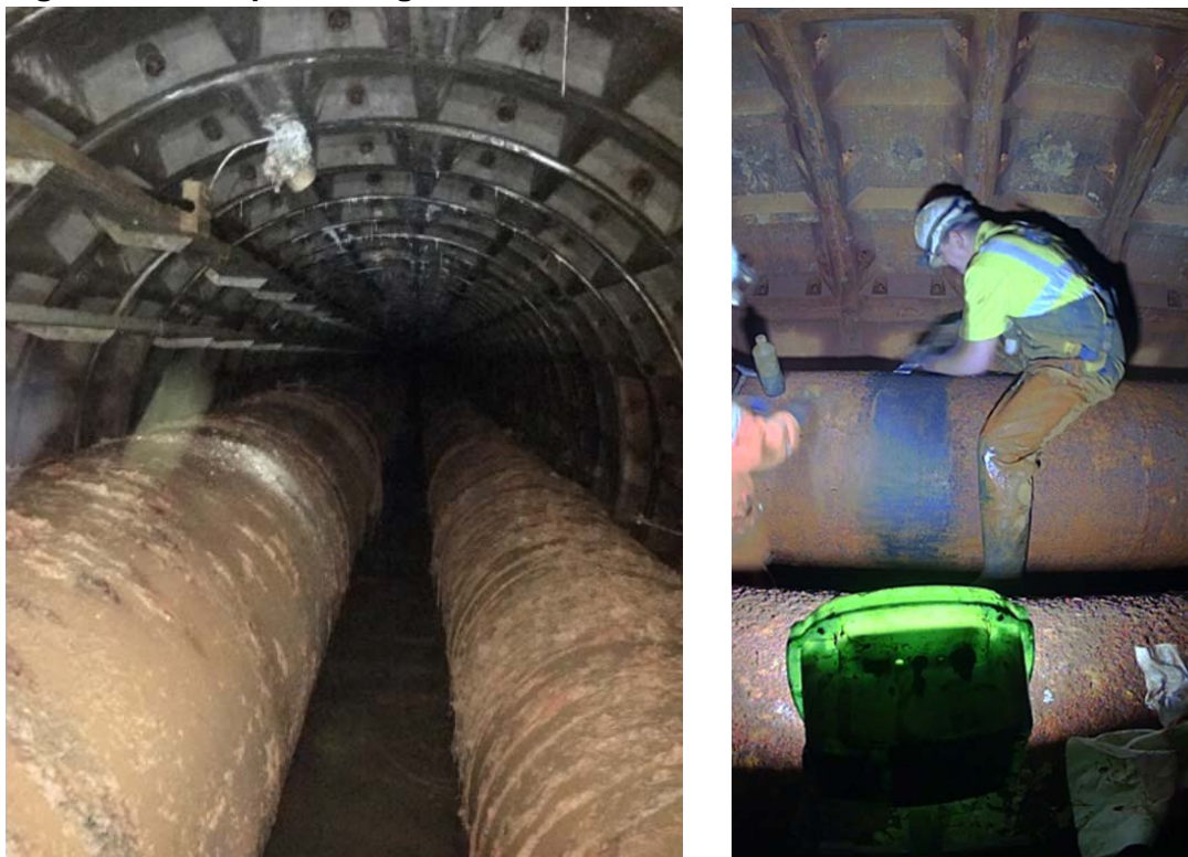
Figure 6-4: Radipole rising mains, located in a tunnel
