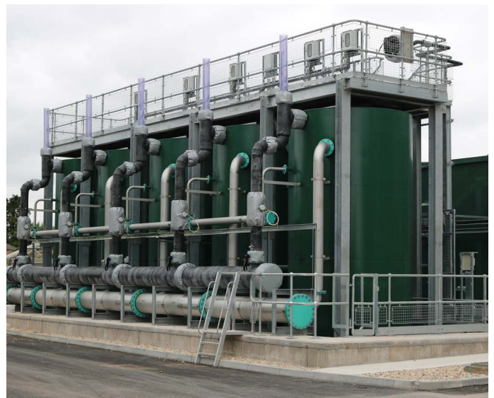
Nitrogen removal plant at Wareham WRC
