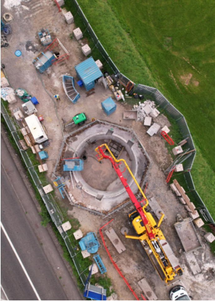
A new below-ground storm tank, capable of holding 125,000 litres of storm water, has been installed in the car park of Bath RFC's rugby ground at Lambridge.
