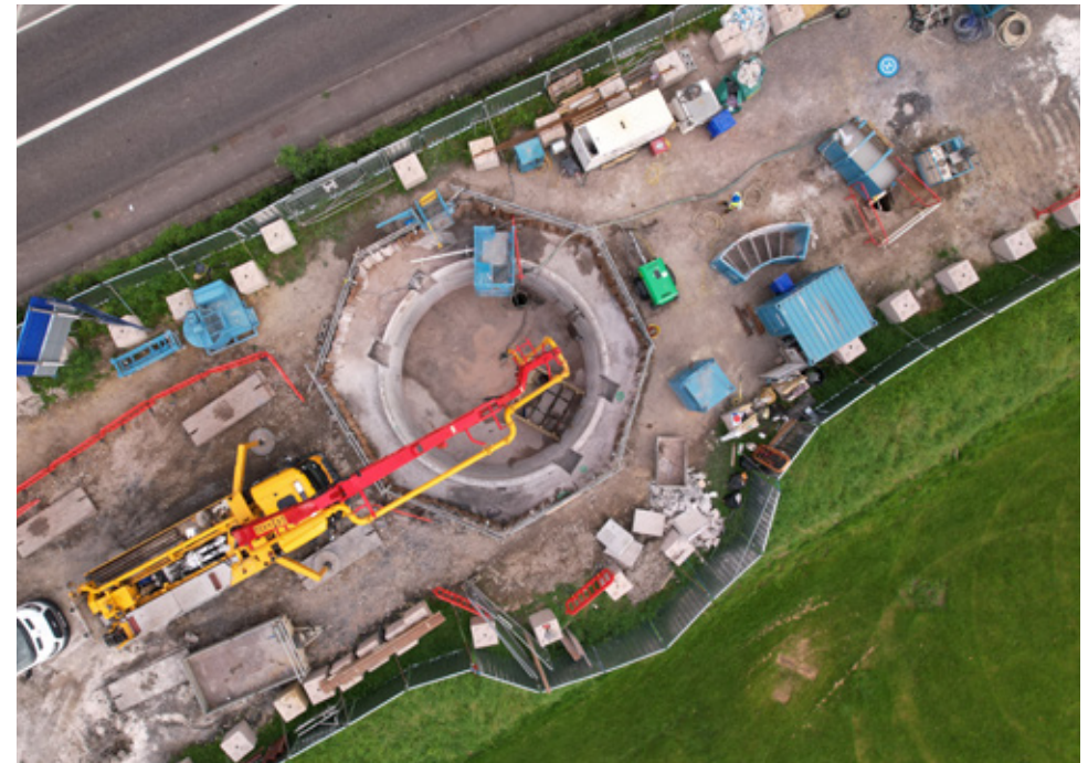
A new below-ground storm tank, capable of holding 125,000 litres of storm water, has been installed in the car park of Bath RFC's rugby ground at Lambridge.
