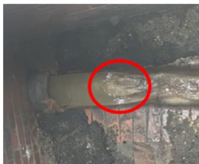
Figure 2: Blockage (circled in red) downstream of the CSO. Note flows are running left to right with high level before the blockage and low fast flows after.
