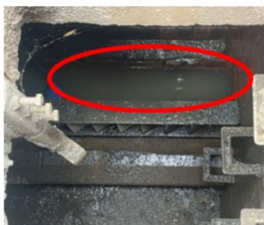
Figure 1: Sewage in the CSO channel flowing slowly (sewage looks still) and at a high level. CSO channel circled in red.
