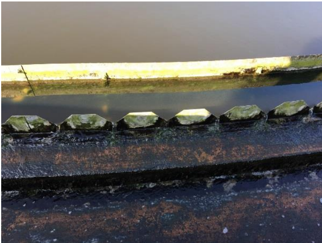
Figure B2: photograph showing pin floc in the final settlement tanks
